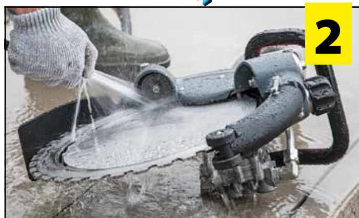
Clean the rollers and housing very carefully with the water hose EVERY DAY after use...
